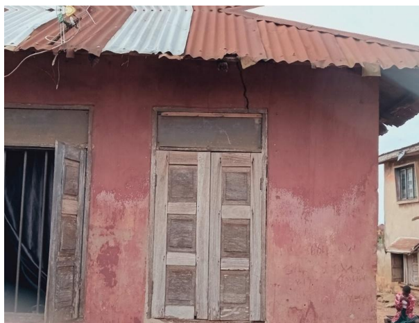
Plate 1: showing a crack on a building in Odopetu District
