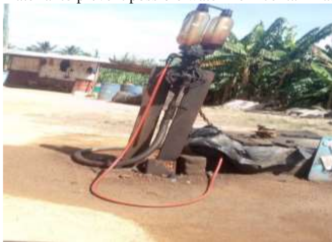
Fig 1 Mechanical Hand Operated Pump station (MHOPSS) Source : (Fieldwork 2017)
